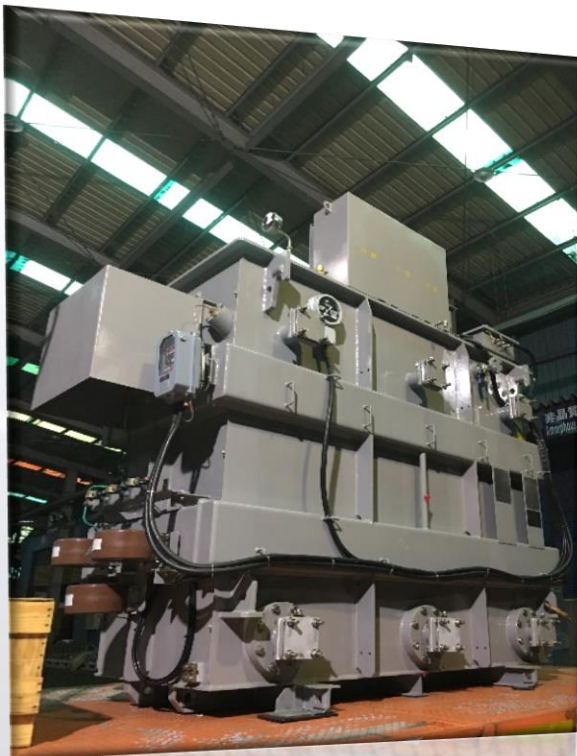
In July 2019, Completion of Hitachi TPC Phase 1 22kV 5.8MW Transformer inside the Wind Turbine Module
