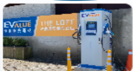
DC Wanli station
