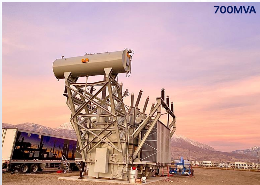
American Northwest Coast 700MVA Super large power transformer
