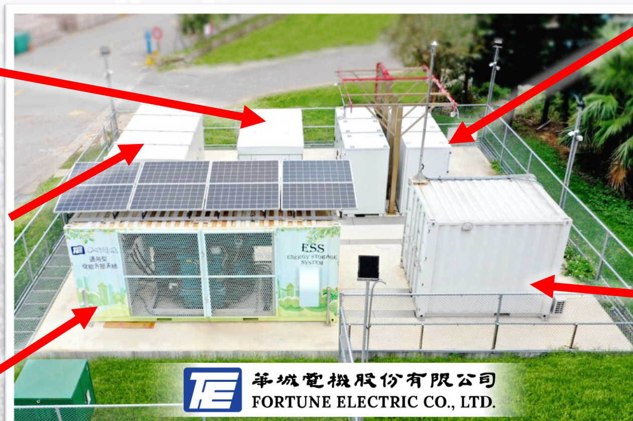
Power Conversion System(PCS)
