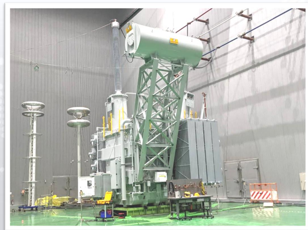
AEP 525kV large power transformer
