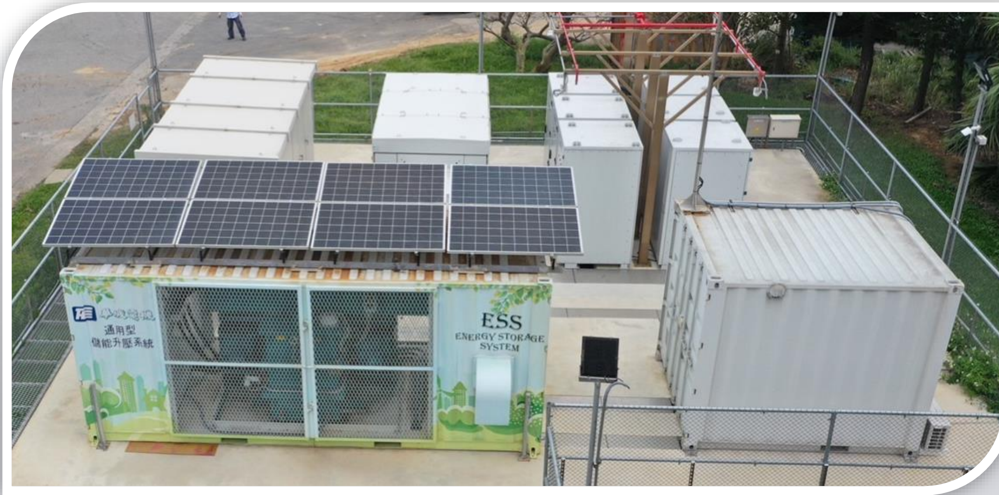
【FE ESS-2MW/2MWh Battery energy storage system demonstration field】
